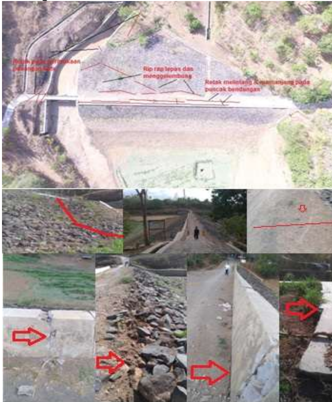
Figure 5 the Gegurik dam after the earthquake
